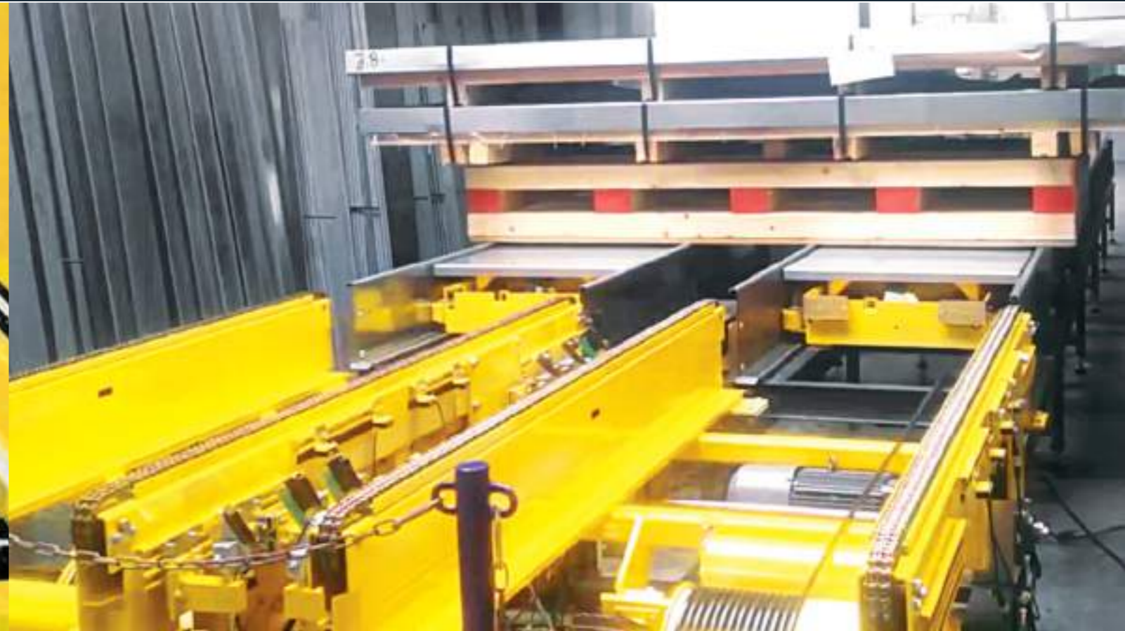
Combination: 2 x 2,5 t Internal transport of sheet metal stack
